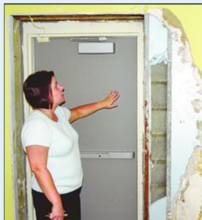
Toni Lloyd, site coordinator of Warren West Community Health Care Center, inspects a wall Wednesday that was damaged by a leaking roof. The operators of the southwest side center closed the doors last week due to air quality issues spurred by moisture seeping into the building. Tribune Chronicle / Joe Gorman
